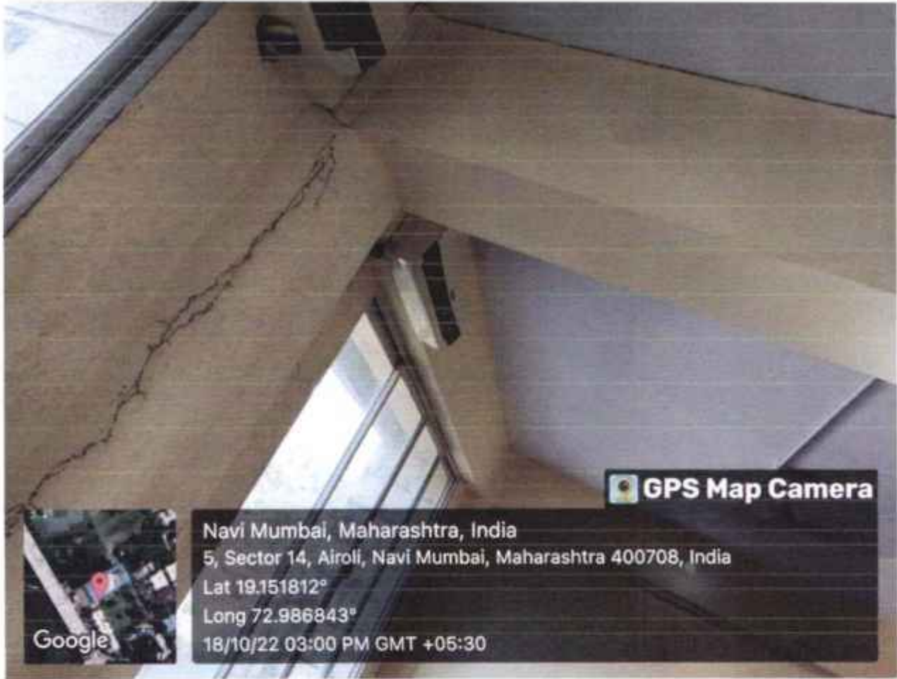
Termite Attack in Classroom No. 106
